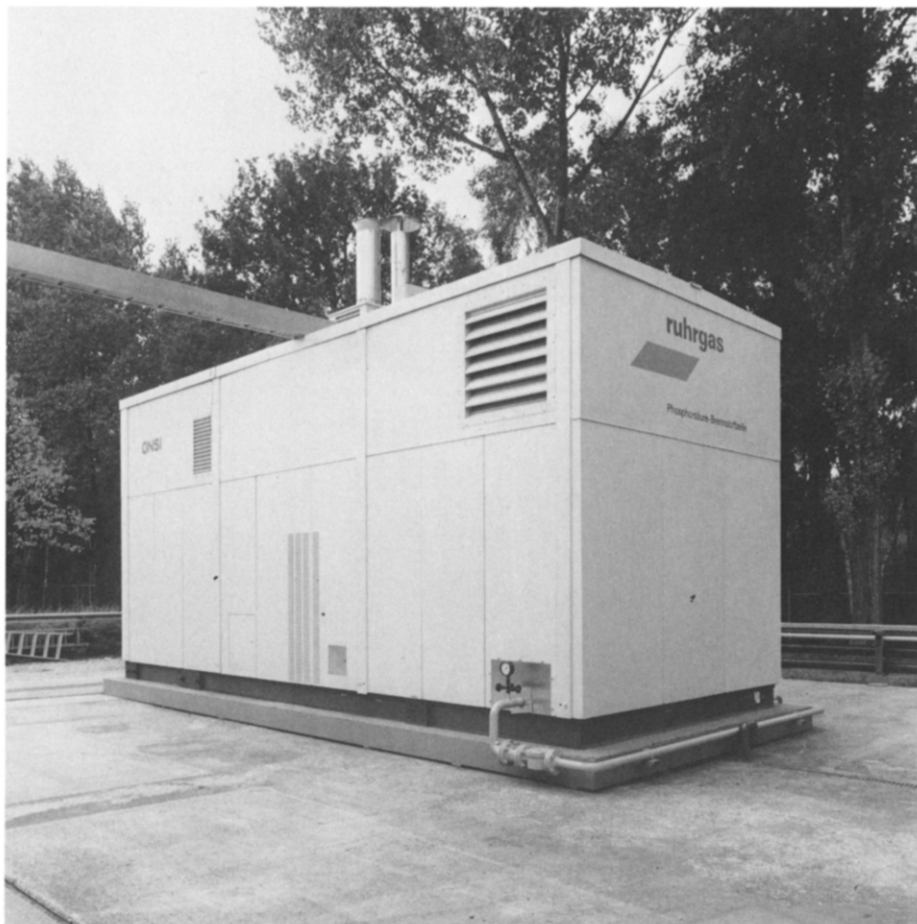
Fig. 3. Installation of the ONSI PC 25 plant at the R&D Facility of Ruhrgas AG, Germany.
